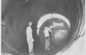
IT SEEMS like an endless operation but sandblasters calmly take it in stride. The interior sections have to be blasted so a gunnite lining can be installed.
